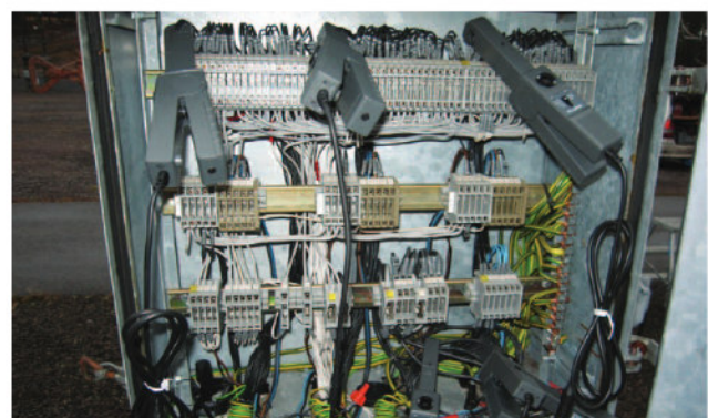
Figure 3. Control cabinet with current clamps
